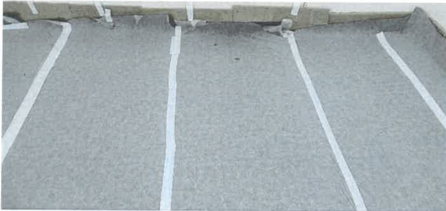
Figure 1: installation situation of impact sound insulating material and edge insulation strips, overlaps with duct tape
